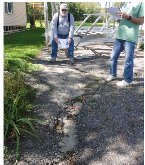
Example of an eroding driveway on the shore of Salmon Lake.
